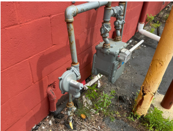
Natural gas line regulator
