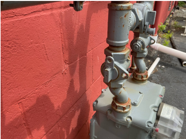
Natural gas supply not shut off, but also not flowing
