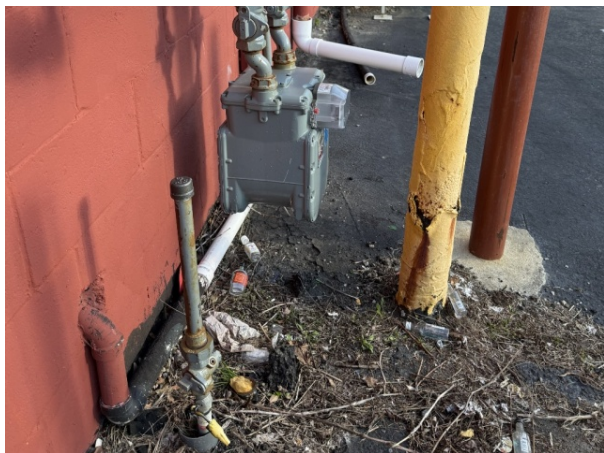
Gas line capped.
